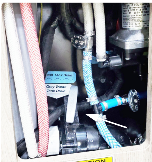
Gray Waste Tank Drain Valve (Located behind passenger rear door below the Water Center Panel. Shown in the closed position- pull out to open T36B shown). - Typical View
