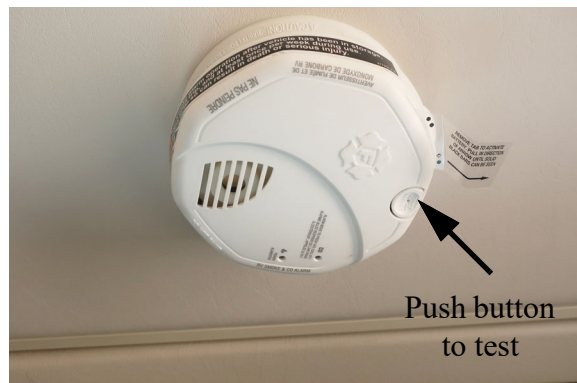
Smoke/carbon monoxide alarm. -Typical View
