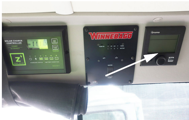
Water heater controls location on Systems Monitor Panel (T36A shown) -Typical View
