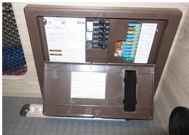
120-Volt Circuit Breakers -Typical View
