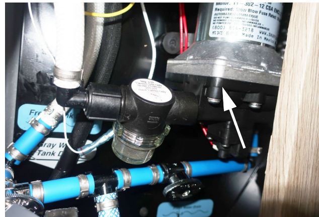
Water Pump Located behind passenger rear door below the Water Center Panel. (T36B shown) -Typical View
