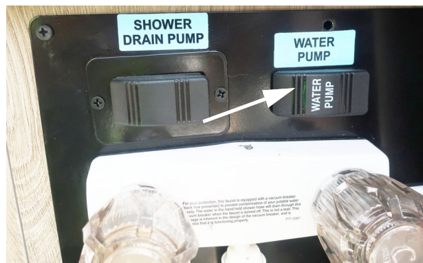
Pump switch T36B -Typical View
