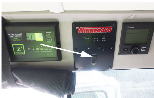
Water pump switch location on Systems Monitor Panel (T36A shown) -Typical View
